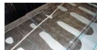
Using vacuum infusion more than halves the amount of resin required, saving almost one tonne on a 45ft catamaran
