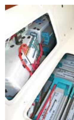
Six converters – one each for the six propulsion batteries in series
