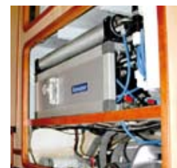
The Schenker watermaker is fitted below the boat's diesel generator
