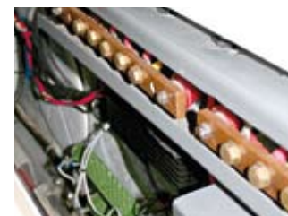
The bus bars will be downsized. The green dump resistors dissipate excess power
