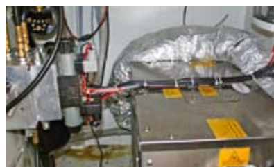
Green eMotion also has an air conditioning unit
